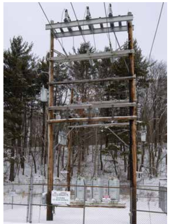
BANDO SUBSTATION: Located along the Mud Pike near the intersection of the Water Level, this historical substation, the Bando Substation, was the first delivery point to members of Somerset REC in 1939. It currently serves 276 members.
