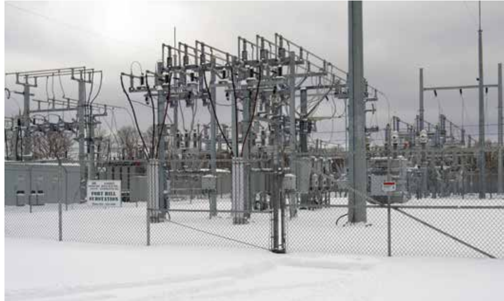
FORT HILL SUBSTATION: Constructed in 2016, the Fort Hill Substation is the most recent addition to Somerset REC’s service territory. It currently serves 2,692 members.
