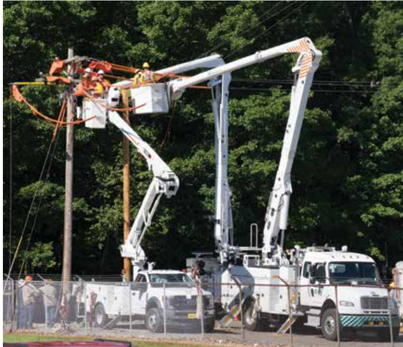
SAFETY FIRST: Somerset REC is a host cooperative for some of the Pennsylvania Rural Electric Association (PREA) training courses. In June, four training weeks were held for employees of Pennsylvania and New Jersey rural electric cooperatives. These training weeks included Basic Rubber Glove, Intermediate Rubber Glove, Basic Hot Stick and Intermediate Hot Stick. Carter Engleka, an apprentice lineman at Somerset REC, participated in Basic and Intermediate Hot Stick training.
